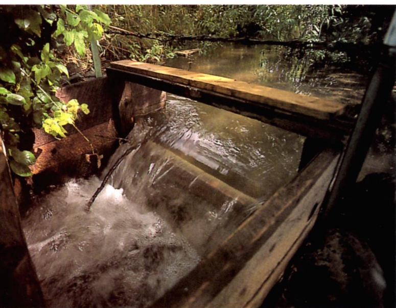
A head gate on the Acequia Madre del Rio Lucero. By taking the boards on top of the gate and inserting them into the stream, farmers can divert the water to a lateral canal.
